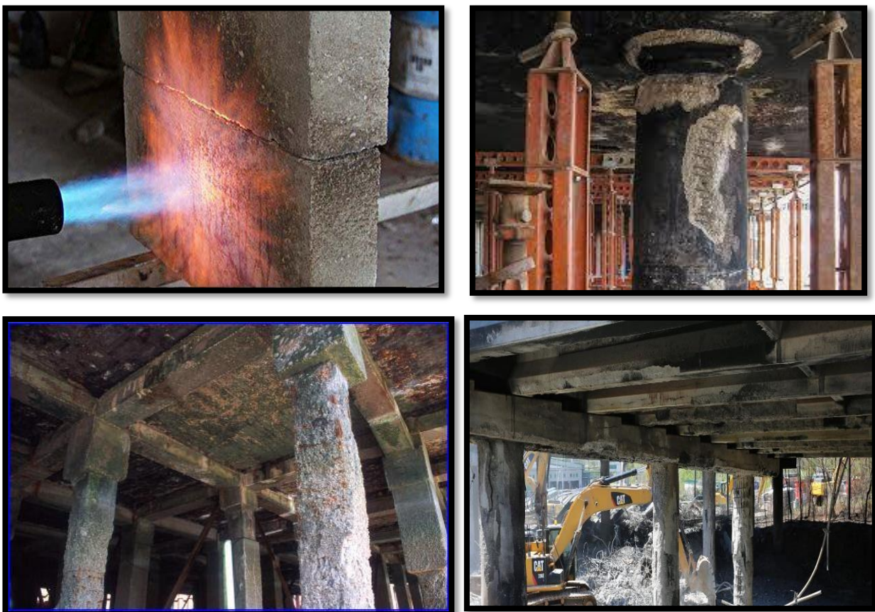
Fig 1.17: Fire damage on concrete structure
