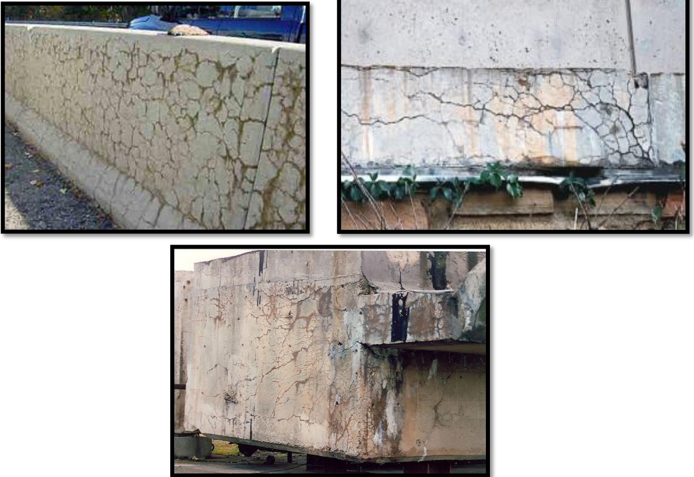
Fig 1.19: Alkali silica reaction on concrete
