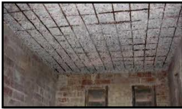
Fig 1.1: Deterioration of Concrete Structures
