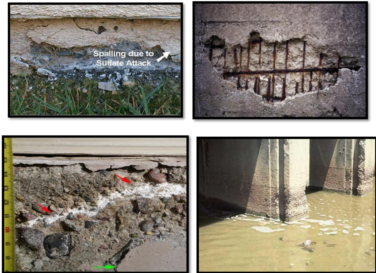
Fig 1.21: Sulphate attack on concrete
